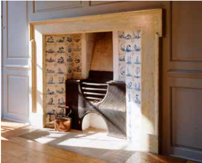
Figure 3 (above) An 18th century cast iron grate in a fireplace at the Great Yarmouth Row Houses.
